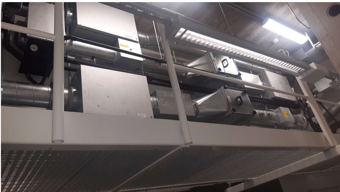
Fig. 5. The thermal conditions and air quality is controlled by two independent ventilation systems for rooms 1 and 2. They are located in the ceiling of the control room.
