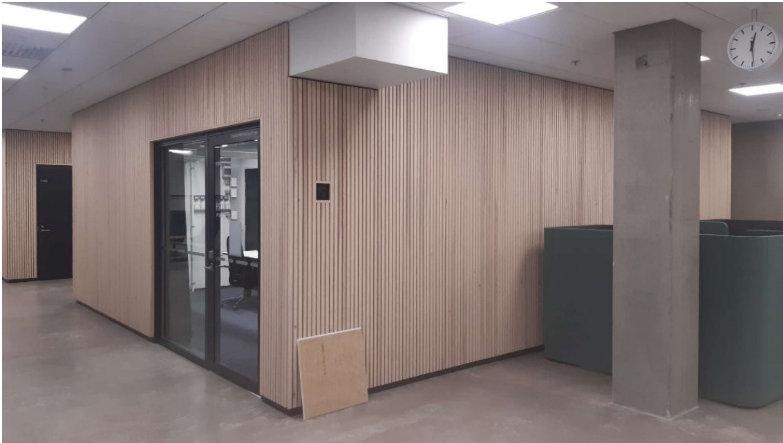
Fig 2. The compartment seen from the outside.
